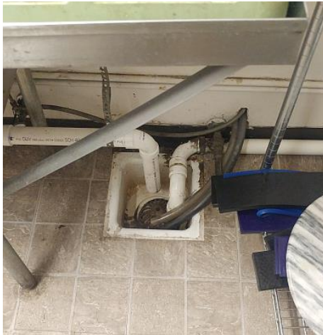
All sinks drain to a proper floor trap.
