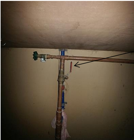
Main water shutoff is where indicated.
