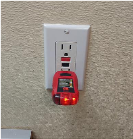
Proper GFCI outlet installed.
