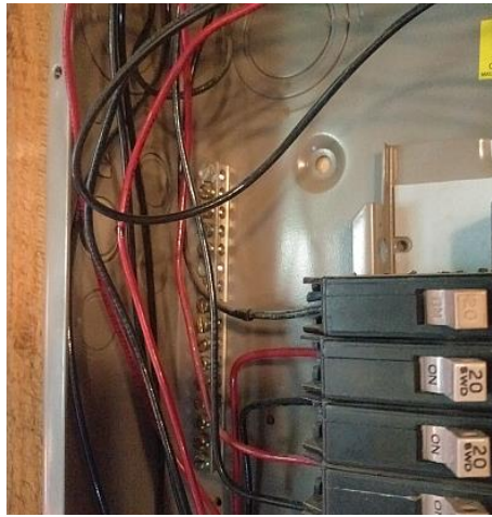
There is no obvious ground. This is a potential Safety Hazard. Recommend Repair.
