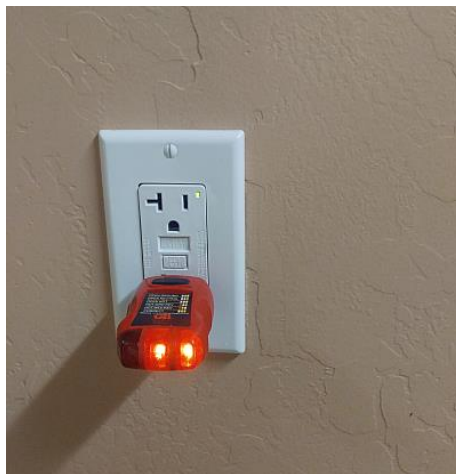
Proper GFCI installed.
