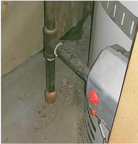
Proper sediment trap installed.
