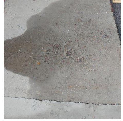
Scaling (loss of surface aggregate) observed. Repair would be cosmetic.
