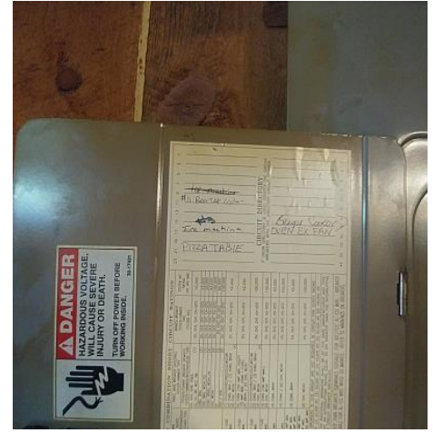
The panel is not completely labeled. Recommend Repair.
