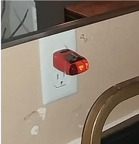
All outlets tested are Proper GFCI.
