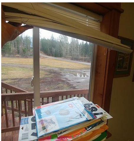
The window screen is not installed. Recommend Replacement.
