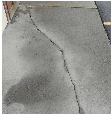
Large settling cracks on service walks. Recommend sealing to help prevent moisture intrusion.
