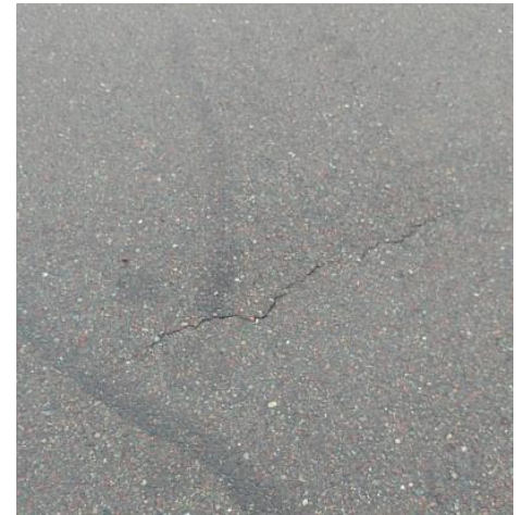
Typical cracks on driveway. No indication of recent movement, no trip hazard.
