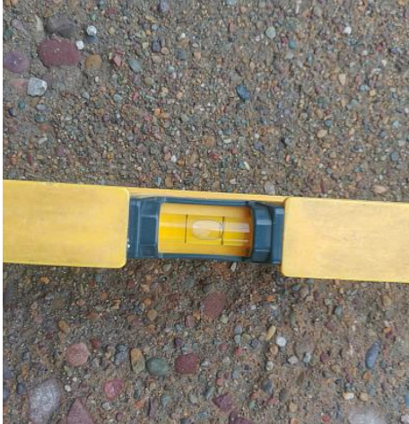
The service walks are pitched toward the building. Recommend Repair.
