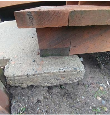
Proper treated wood used for contact with concrete. Material has eroded from under the concrete pad the steps are resting on. Recommend Repair (backfill).
