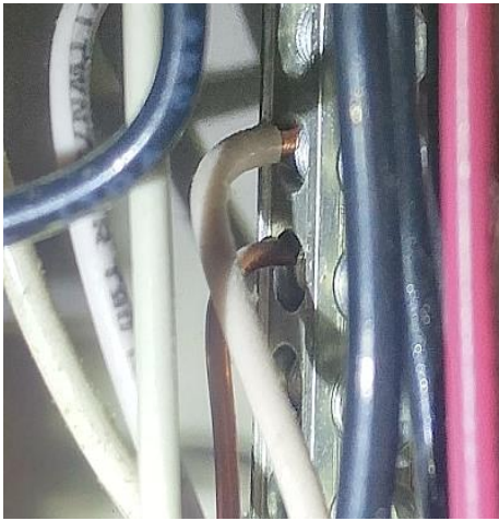
The neutrals and grounds are not isolated. This is a potential Safety Hazard. Recommend Repair.
