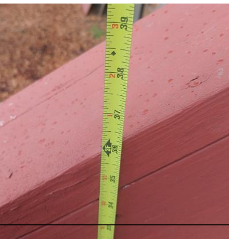
The railing is the proper height.
