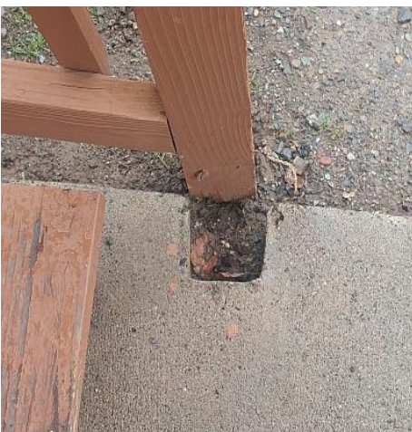
The rail post has deteriorated and is loose. The loose railing is a potential Safety Hazard. Recommend Repair/Replacement.
