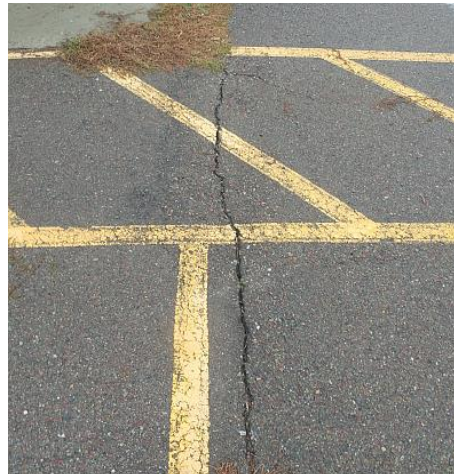
Large settling cracks on the driveway. Recommend sealing to help prevent moisture intrusion.
