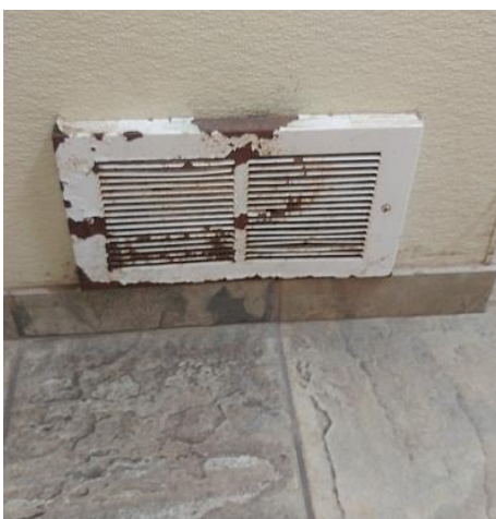
The in wall electric heater is not operating. The cover is rusted. There is no visible thermostat for the heater. Recommend Repair/Replacement.
