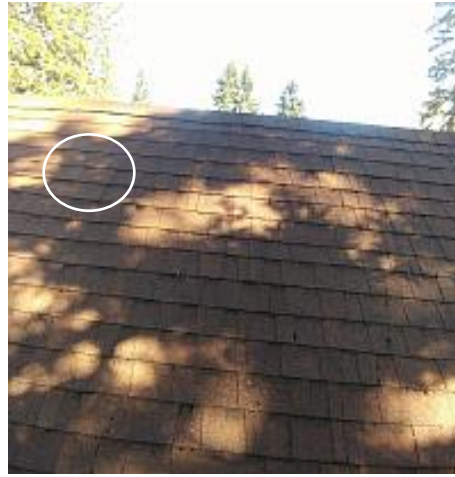
Slight 'bow' observed in the roof cover in one area (not really visible in the photo). Cause unknown. Recommend Repair.
