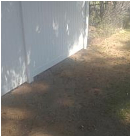
Indications of leaking insulated glass observed. Recommend Replacement.
