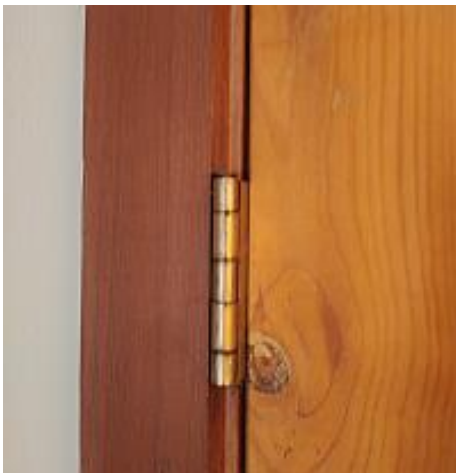
The upper hinge squeaks. Recommend Repair (lubrication).
