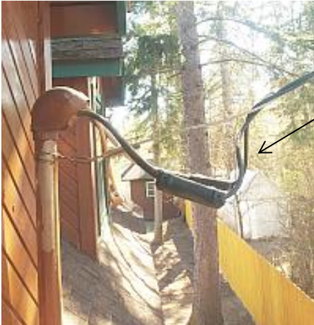
The drip loop is not properly installed. The drip loop should channel runoff away from the splices. Recommend Repair.
