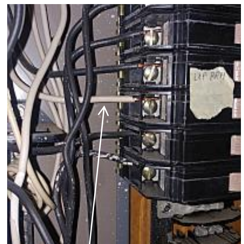
White (neutral) wires used as black (live or line) wires should be color coded black or red with electricians tape.
