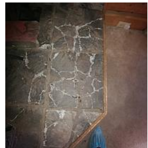
Cracked/loose hearth stones observed. Recommend Replacement.
