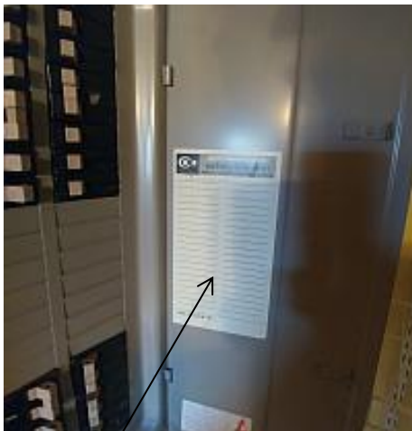
The breakers are not labeled. Recommend Repair.
