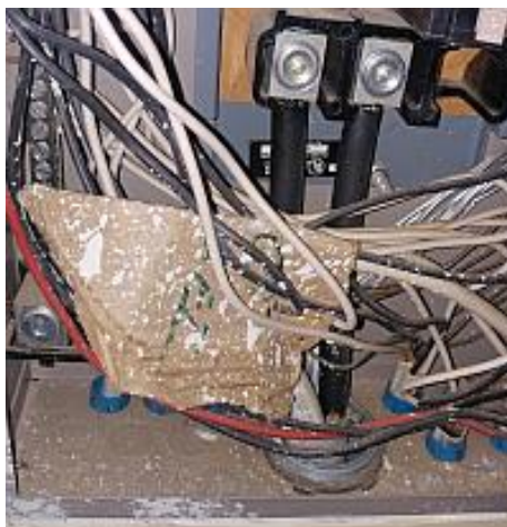
A piece of cardboard is being used to label a wire. There are (nonflammable) products designed specifically for this. Recommend
