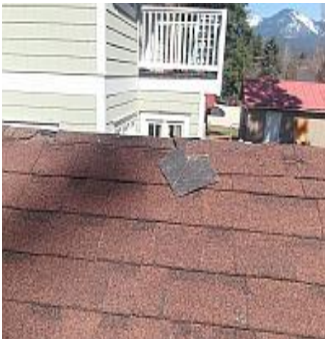
Missing/damaged shingles observed. Recommend Repair/Replacement.
