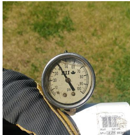
The water pressure is 40psi, which is within acceptable limits.
