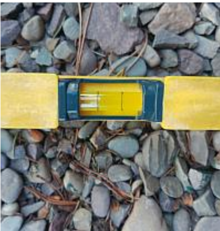
The driveway is pitched toward the home. Recommend Repair.
