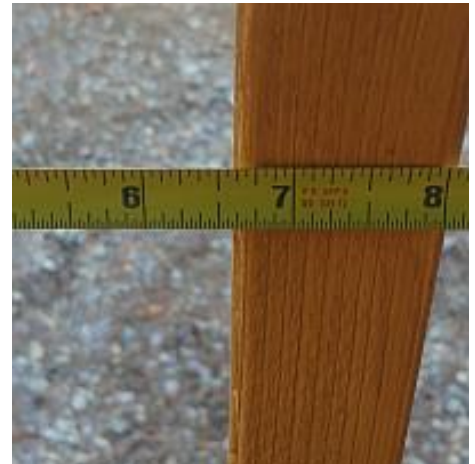
Balusters are improperly spaced. Recommend Repair.
