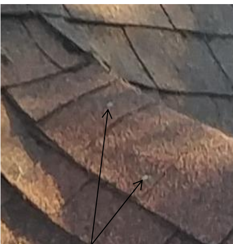
Exposed nail heads observed. Recommend sealing to help prevent moisture intrusion.
