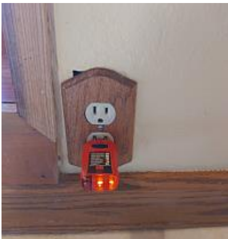
The kitchen outlets are not GFCI. While required by current standards, this home was constructed before those standards were in place. It is highly recommended that all kitchen outlets be GFCI. Recommend Repair/Replacement.
