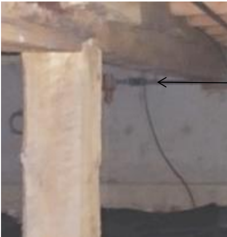
Main water shutoff is in the crawl space where indicated.
