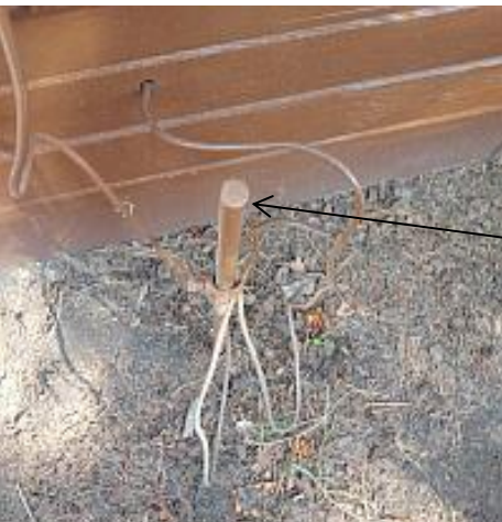
The ground is not proper. All of the grounding rod must be buried. A portion of the grounding rod is visible above ground. This is a Major Concern. Recommend Repair.
