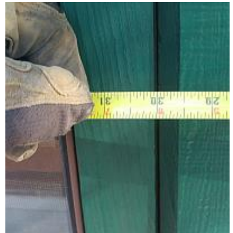
The service mast and conductors are less than 3 feet from an opening window. Overhead service conductors must maintain a clearance of 3 feet from windows that open or similar locations. This is a potential Safety Hazard. Recommend Repair.
