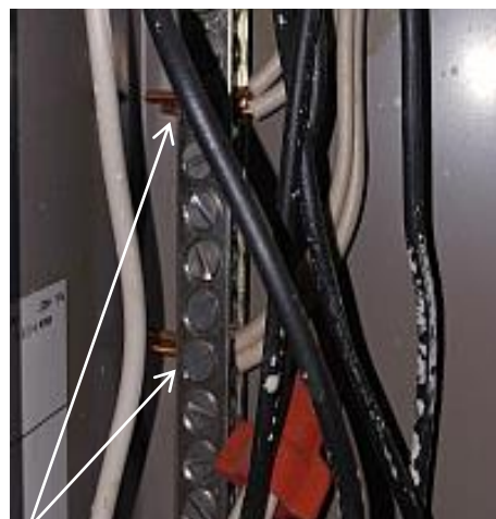
There are numerous double tapped neutral and ground wires. Unless otherwise marked these terminals are designed for one wire per lug. Recommend Repair.
