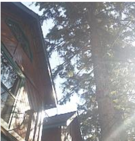
Vegetation in several areas is in direct contact with/overgrowing the home. Recommend Trimming.
