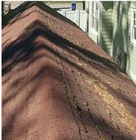
Moss/lichen growth observed. This growth can, over time, deteriorate a roof cover. Recommend Removal.
