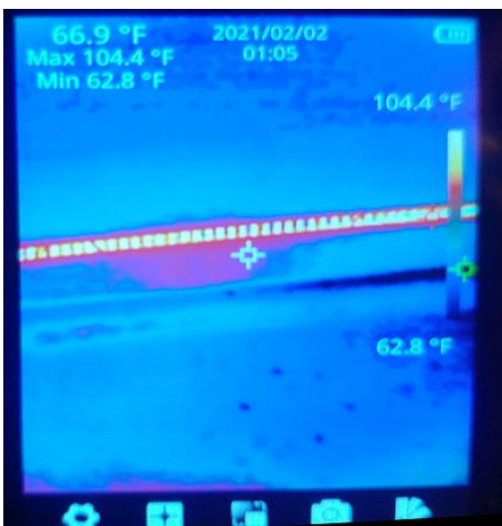
The baseboard electric heater is operating.
