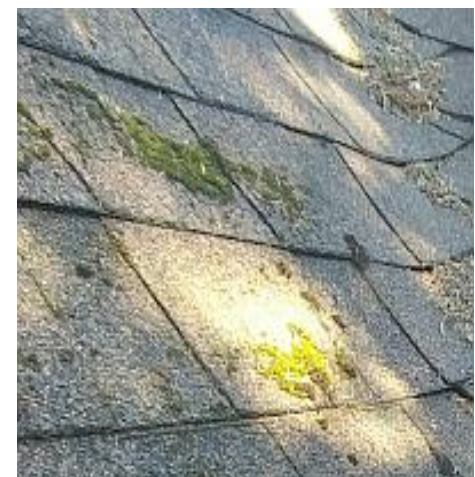
Moss/lichen growth observed. This growth can, over time, deteriorate a roof cover. Recommend Removal.
