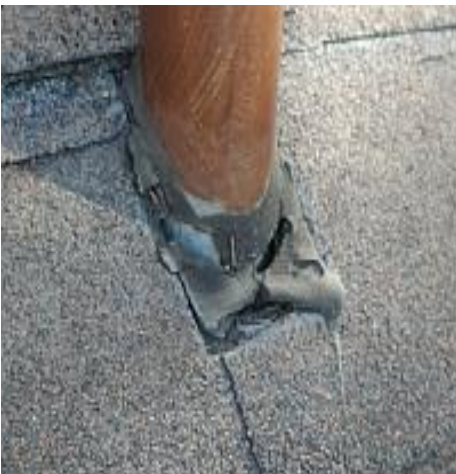
The weather boot is cracked/holed. This is a Major Concern. Recommend Replacement.
