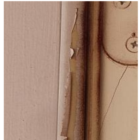
The weather stripping is painted, which causes it to loose flexibility and therefore effectiveness. Recommend Repair/Replacement.
