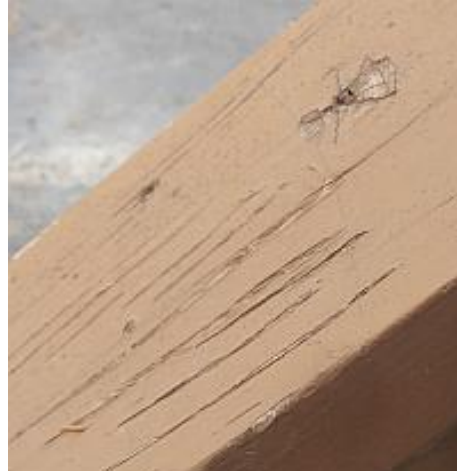
The railings are weathering. Recommend prepping and sealing (painting/staining). Recommend Repair.
