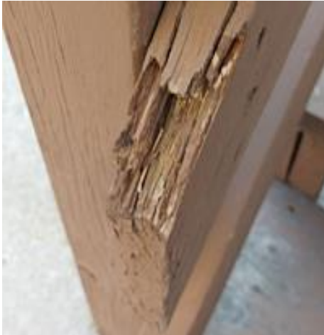
The railing is deteriorated in areas. This is a Major Concern. Recommend Repair/Replacement.
