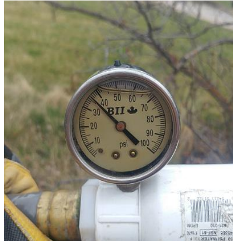
The water pressure is 36psi, which is within acceptable limits.
