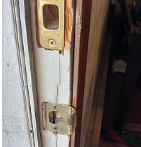
The weather stripping is torn/holed. The door frame is dinged/cracked. Recommend Repair/ Replacement.
