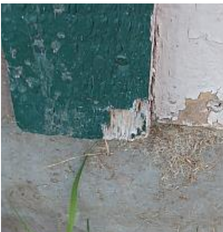
The trim is weathering/slightly damaged. Recommend prepping and sealing (painting/staining). Recommend Repair.
