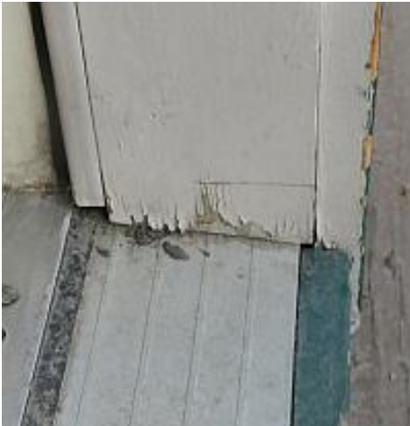
The exterior door frame is weathered. Recommend prepping and sealing (painting/staining). Recommend Repair
