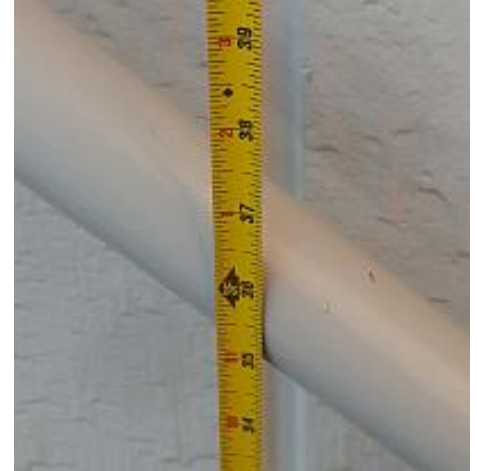
The hand rail is the proper height.
