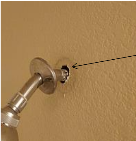
Recommend caulking where indicated to help prevent moisture penetration into the walls.
