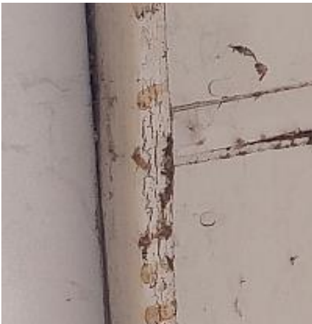
The fascia is weathering. Recommend prepping and sealing (painting/staining). Recommend Repair.
