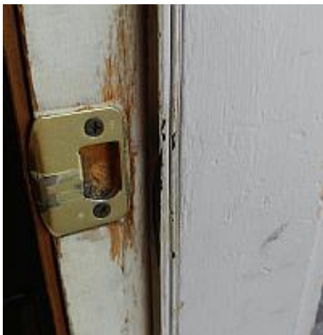
The weather stripping is torn/holed. Recommend Repair/Replacement.
