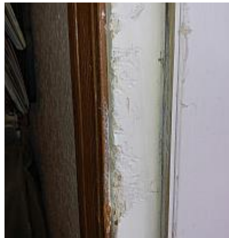
The interior door frame is dinged. Recommend Repair
