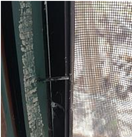
The screen is loose. Recommend Repair.
