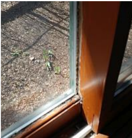
The wood windows are weathered. Recommend Repair.
