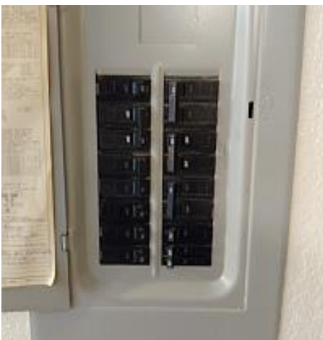
The main panel is in Satisfactory Condition.
