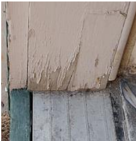
The exterior door frame is weathered. Recommend prepping and sealing (painting/staining). Recommend Repair
