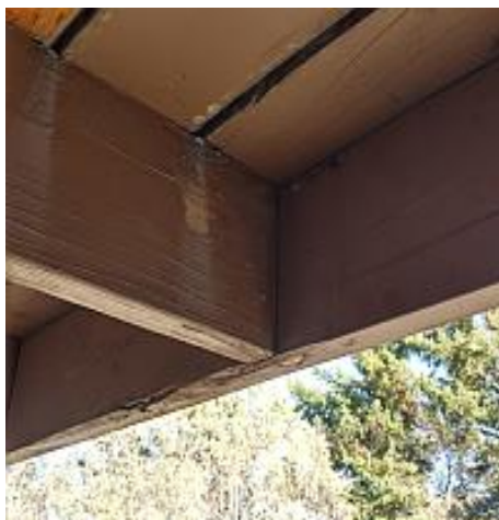
There are no joist hangers installed on the rim joist. Although not specifically required as the rim joists carry little load on a cantilevered deck, the inspector recommends properly installed joist hangers to help ensure positive attachment between the joists and rim joist.
