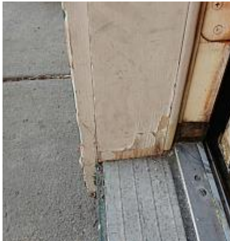
The exterior door frame is weathered. Recommend prepping and sealing (painting/staining). Recommend Repair
