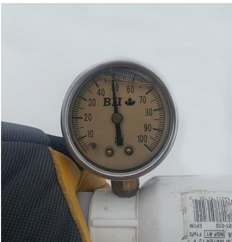
Water pressure is 48psi, which is within acceptable limits.
