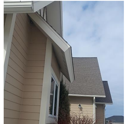
The gutters are not completely installed. Gutters help divert runoff away from the foundation and help keep backsplash away from the homes siding. Recommend Replacement.
