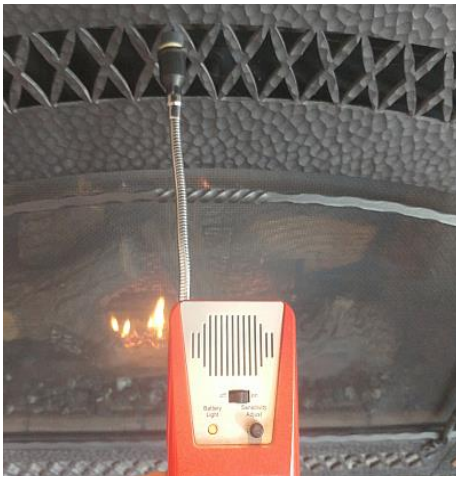
No gas or CO leaks detected. Testers TIF 8800/DCO 1001.
