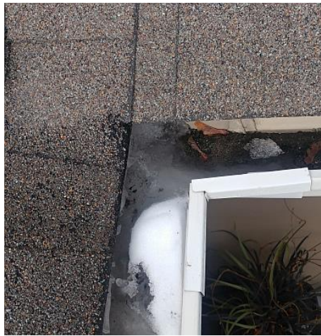
The gutters are dirty. Recommend Cleaning and seasonal cleaning thereafter.
