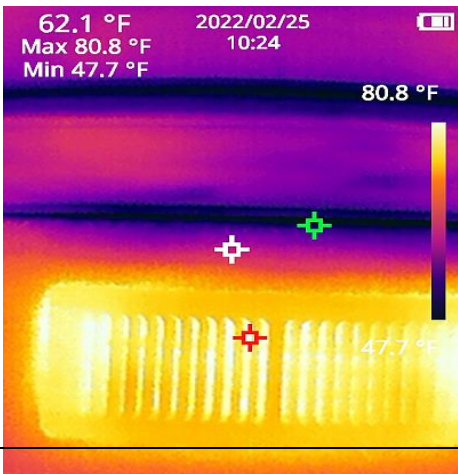
The register is in Satisfactory Condition. The in floor hydronic heating system is operating.
