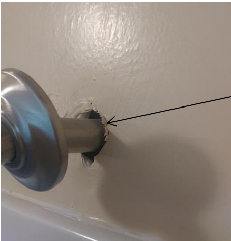
Recommend caulking where indicated to help prevent moisture penetration into the walls.
