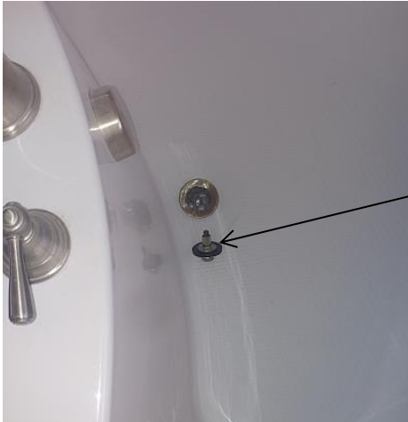
The built in stopper is not installed.
