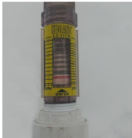
Water pressure is 9psi, which is within acceptable limits.
