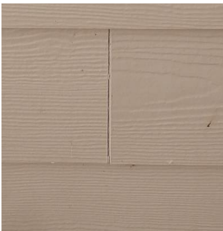
Calking needed on numerous siding joints. Recommend Repair.
